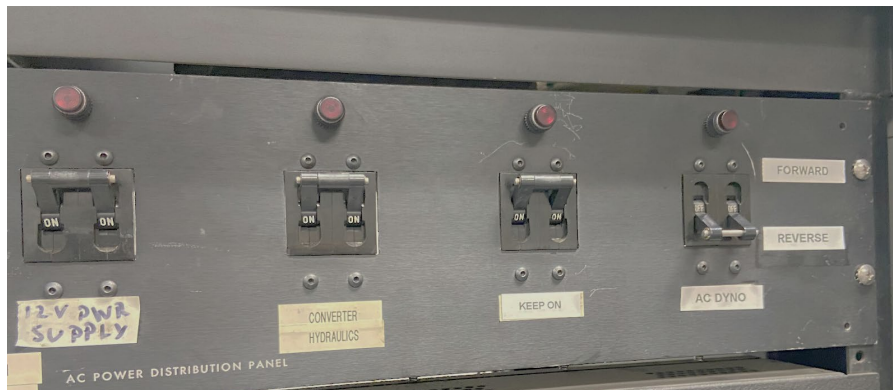
Figure 24: AC Dynamometer direction set to FORWARD
