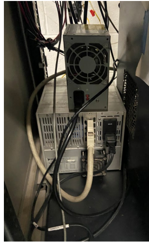
Figure 25: NI Controller box
