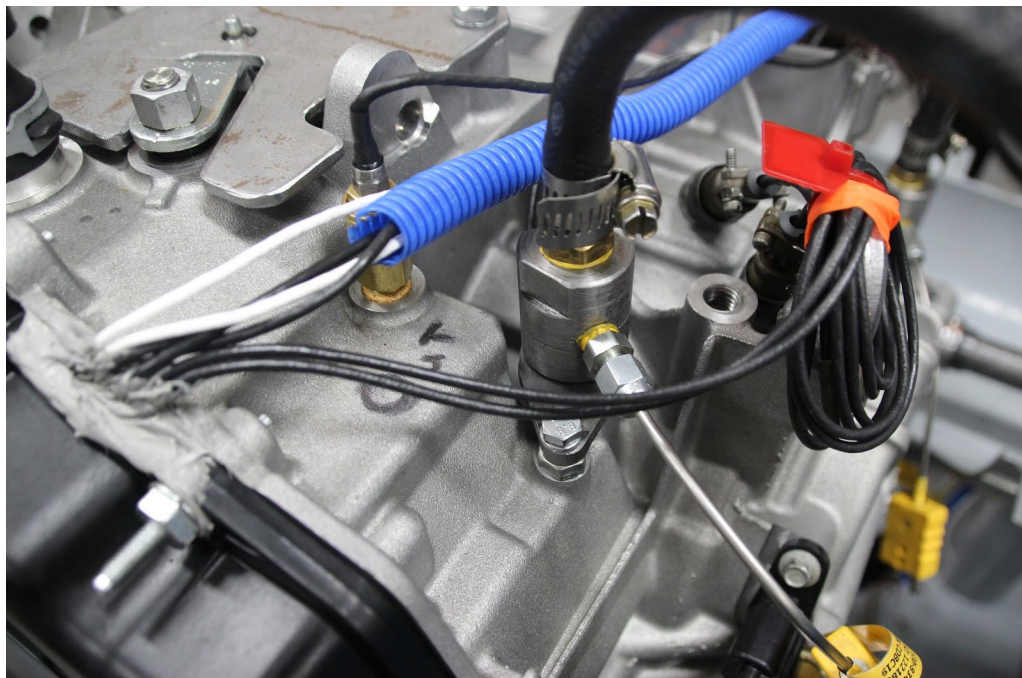
Figure 135: Outlet transmission ATF line
