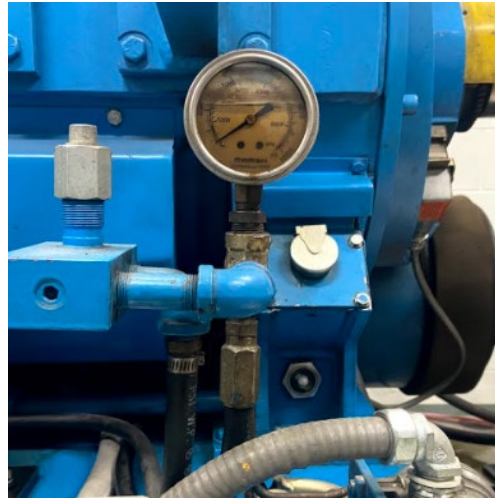
Figure 53: Oil pressure gauge for AC dynamometer bearings
