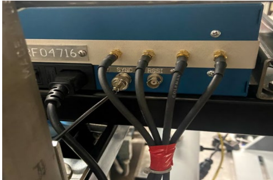
Figure 41: Four antennae connections for Transmitter C – red
