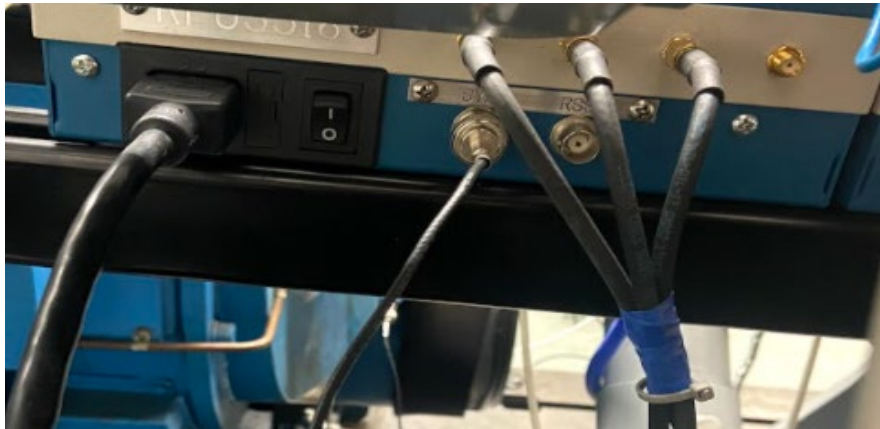
Figure 39: Three antennae connections for Transmitter B – blue
