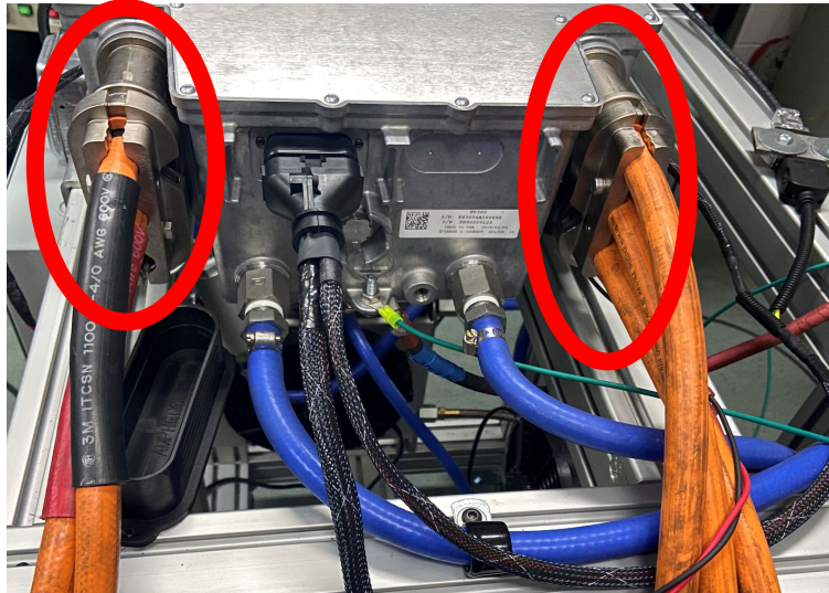
Figure 35: High current connections to the inverter cart. On the left, DC power from the dynamometer cabinet, and on the right, high current AC power feeding the e-motor.
