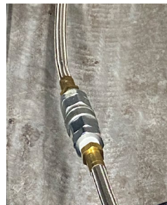
Figure 33: Cooling line connection for electric motor to inverter cart cooling system
